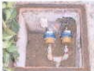
Example of a Waveflow installed and plugged to 2 water meters.
